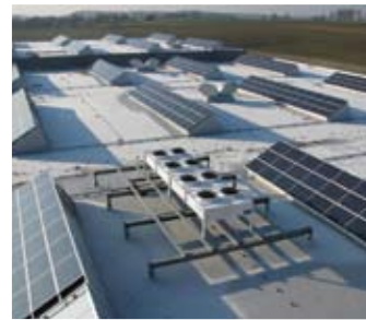
From left to right: Heating room with heat pump, compressor unit with heat recovery system, photovoltaic system and heat exchanger for discharging excess heat.
