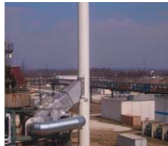
From left to right: Corporate Centre of Evonik Industries AG in Essen, implementation of agreed measures by the team, thermal post combustion flue gas chimney with upstream heat exchanger for boiler feed water preheating.
